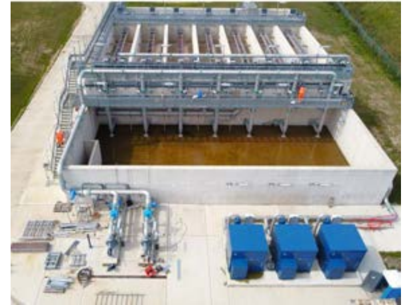
Scaynes Hill Deep bed sand filter in commissioning
