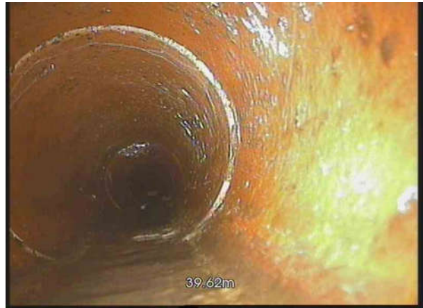
2, 00:03:30, 39.62 m Crack, circumferential at joint from 10 o'clock to 02 o'clock
