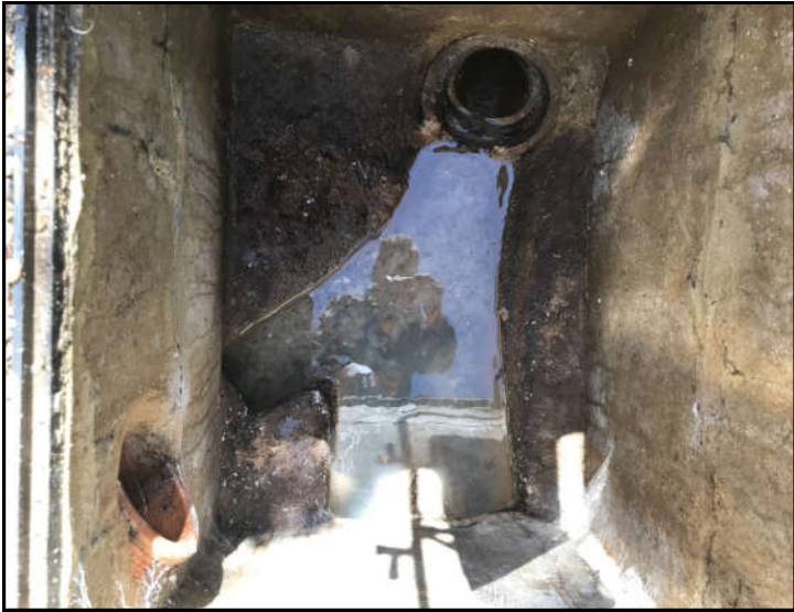
IC1 - BLOCKED AT TIME OF SURVEY
